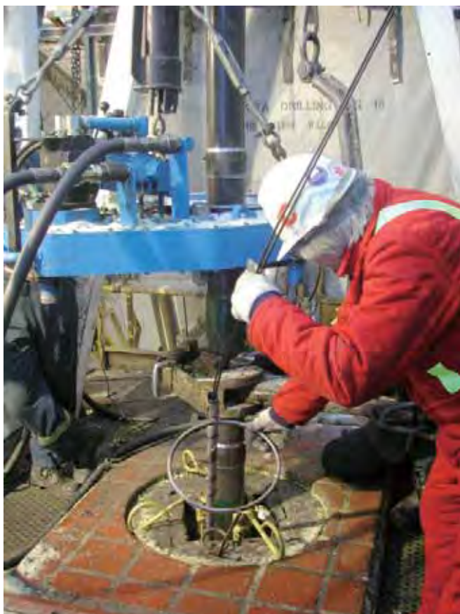
Figure 1. Distributed Temperature Profiling (DTS) fiber-optic cable installation for permanent temperature surveys behind the casing at Mallik Gas Hydrate drilling site in Canada. Fiber-optic cables are attached to the outside of the casing wall by special cable clamps to prevent cable damage while running into the hole. Special cable outlet connectors at the well head ensure safe data retrieval from the cemented borehole annulus to the surface.
