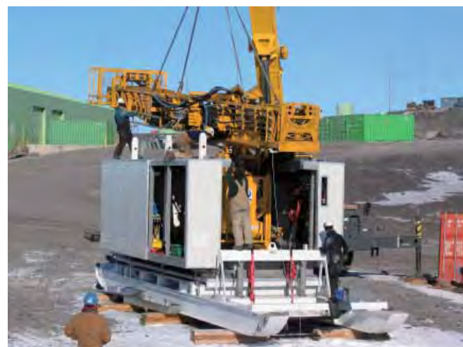
Figure 3. Attaching drilling rig mast to jack-up platform after off-load in McMurdo. Assembly of ANDRILL System at ice edge near New Zealand's Scott Base.
