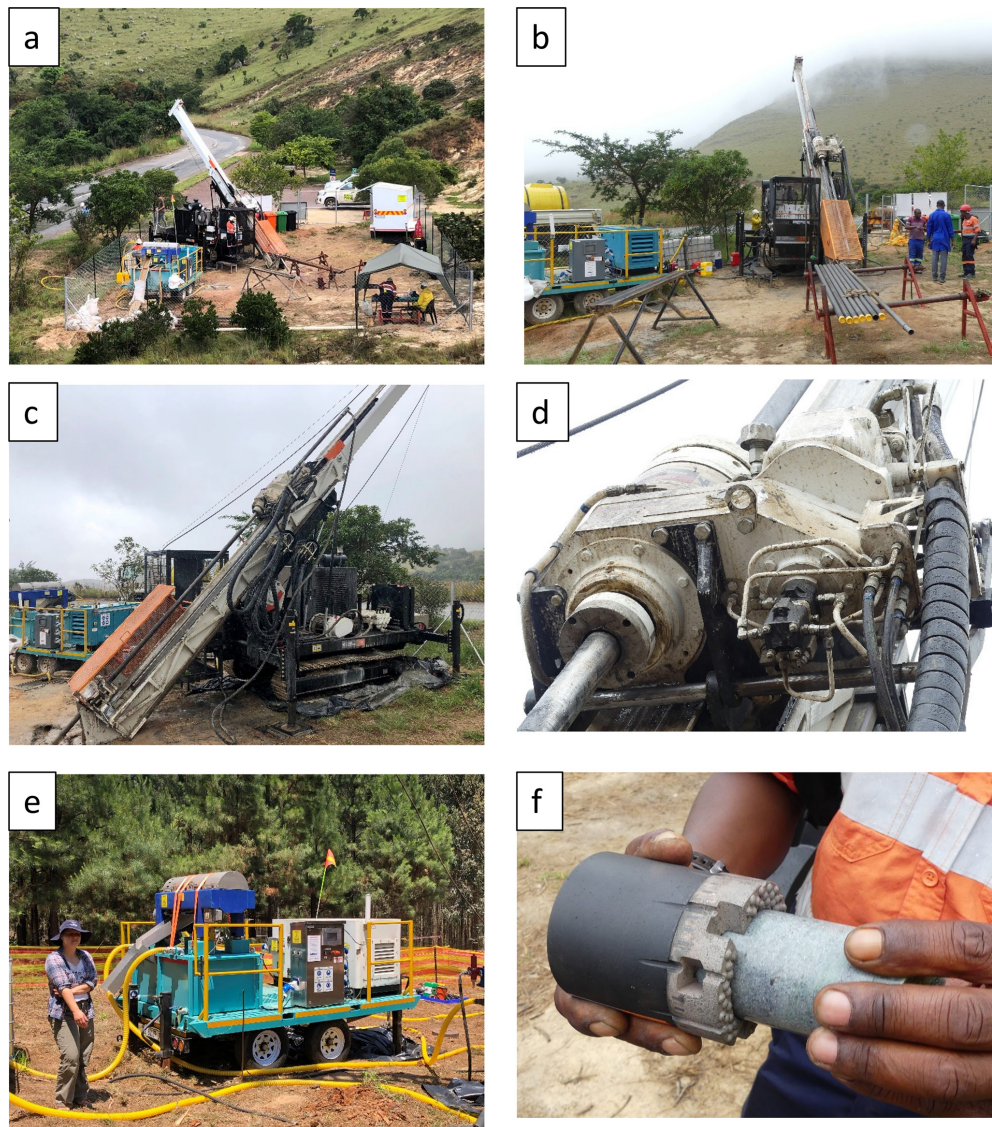
Figure 7. Drilling setup at Site 2. (a) Overview of the site: from left, bagged sludge, trailer-mounted Solid Removal Unit (SRU), drill rig MDX317, and the tressels and workbench for the drill pipes, tented work area, and storage trailer. The entire site is fenced. (b) Site overview. (c) Track-mounted drill rig. (d) “Top drive”. (e) SRU. (f) Rotary drill bit with a piece of core.
